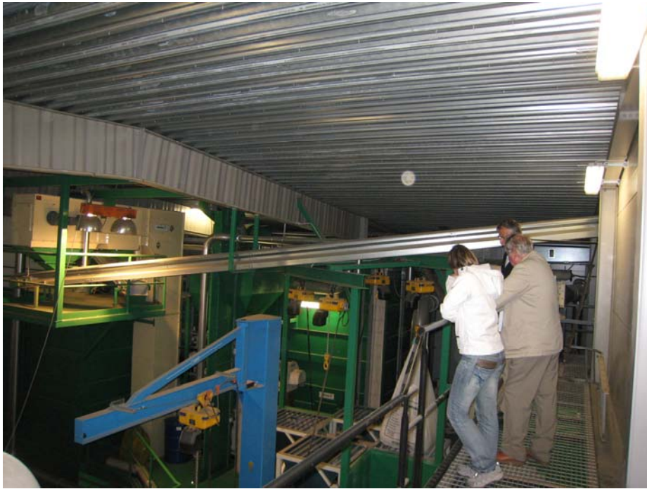
From the study visit platform visitors get a top view of the facility.
