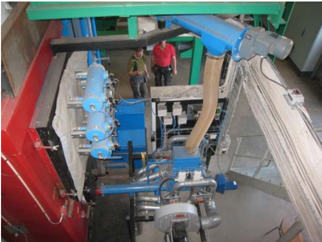
1250 BIOAGRO Boiler with automatic sooting system – view from first level audience platform.
